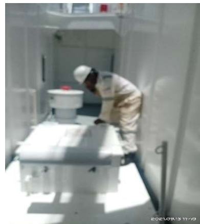
Ventilation closed by 4EO & Oiler
