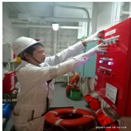
CEO releasing water mist system manually.
