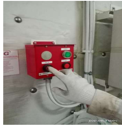
Emergency stop button for pumps and blower operated.
