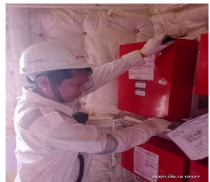
CO2 cabinet opened and operate control valve for main and to bottles.
