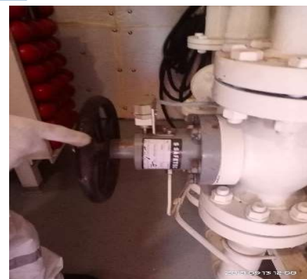
Confirm CO2 main valve open
