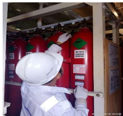
Confirm 95 bottles of CO2 valve activated. 95 Bottles hose were cold.
